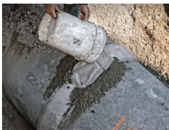
Grout is poured into the diaper into one side and then the other until the diaper is completely full
