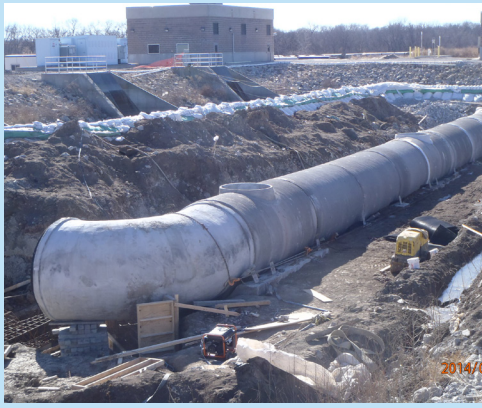
Piers assure Concrete Pressure Pipe laid in unstable soil will maintain the required elevation after soil settlement.
