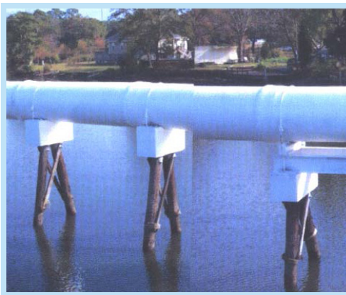
Concrete Pressure Pipe river crossing.
