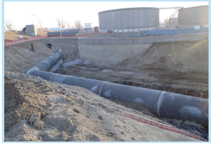
Concrete Pressure Pipe in sewage treatment plant.
