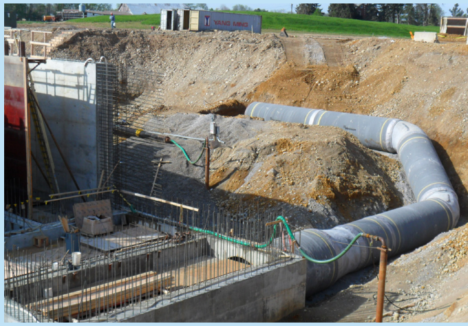
Concrete Pressure Pipe in sewage treatment plant.
