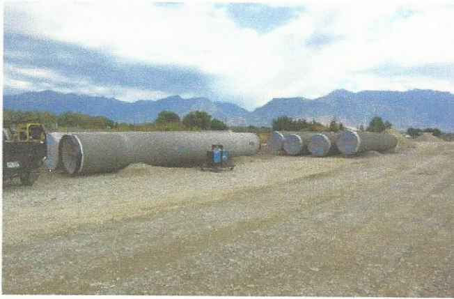
ABOVE ▲ Since minor corrosion and mill scale won't affect the passivation properties of mortar coatings, abrasive cleaning and surface profiles are not required prior to installation.
