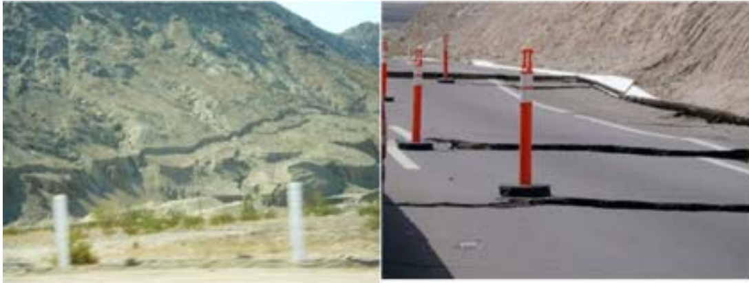
Figure 7. Extensive Damage (right picture) to the Mexicali-to-Tijuana Highway at kilometer 20 at the Laguna Salada Fault Crossing. The Fault line can be observed in the left picture.
