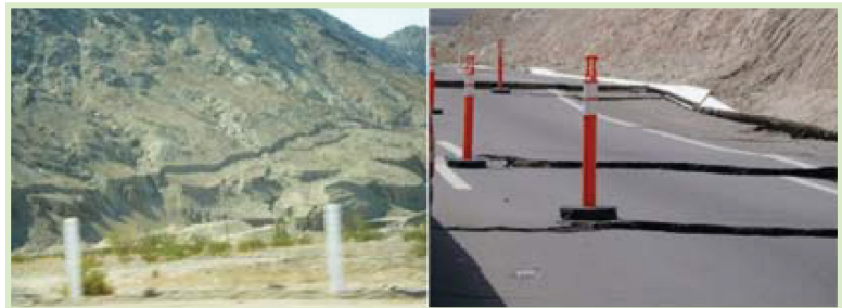
Figure 1. Extensive damage (right picture) to the Mexicali-to-Tijuana Highway at kilometer 20 at the Laguna Salada Fault Crossing. The fault line can be observed in the left picture. A 60" PCCP line with gasketed joints is installed parallel to this highway. The PCCP was inspected by potholing several locations and found to be undamaged.
