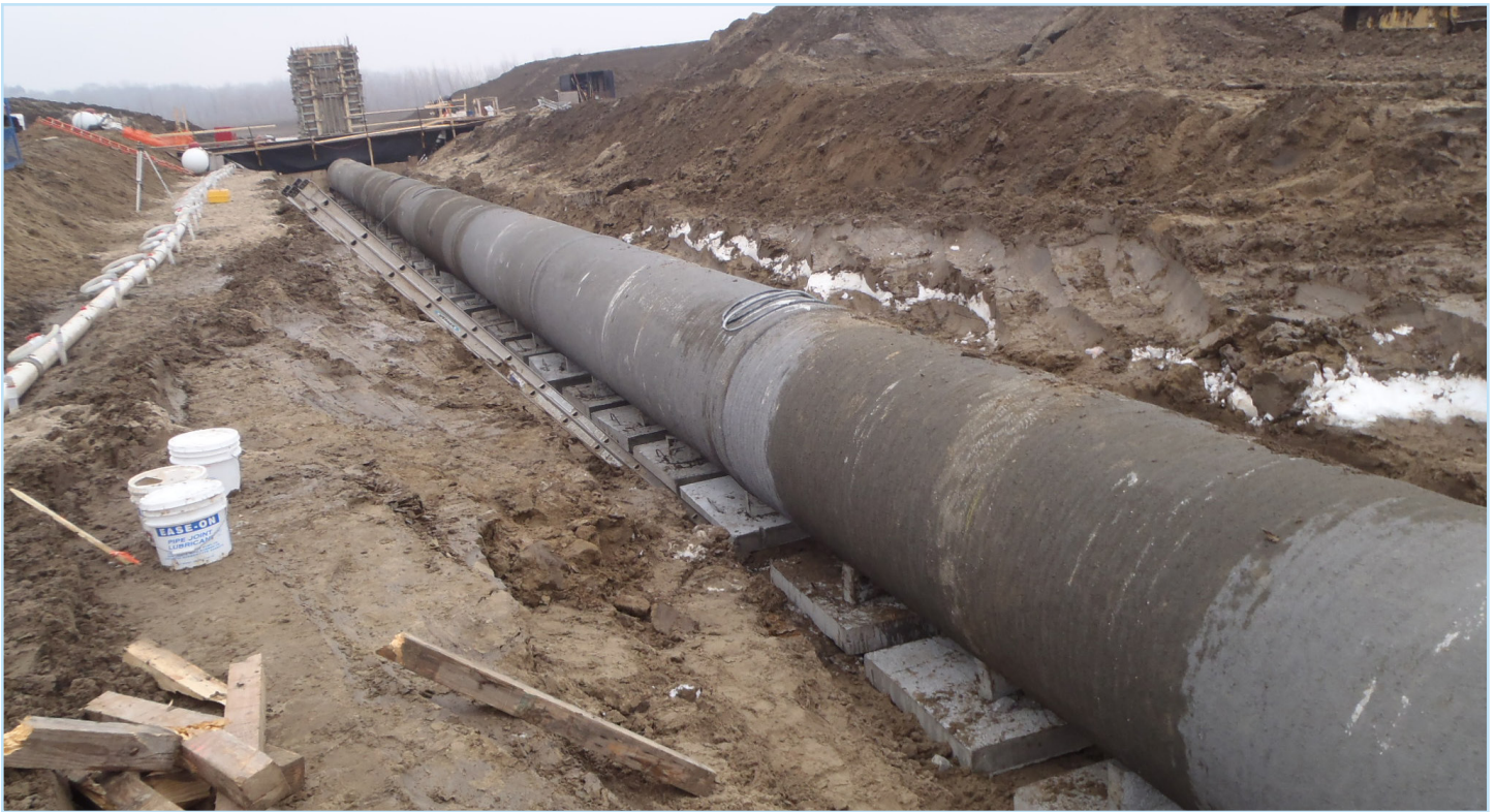
Principal spillway of concrete pressure pipe laid to grade, with forming for vertical intake structure in background.
