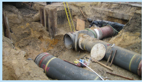
Chilled water lines being installed for the University of Wisconsin, in Madison, WI
