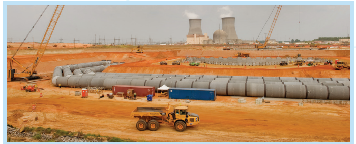
Southern Company's Vogtle Units 3 & 4 in Georgia are the first new generation nuclear plants in the US. The circulating water system includes more than 12,000 feet of Concrete Pressure Pipe carrying water from the turbines to the cooling towers and back again.
