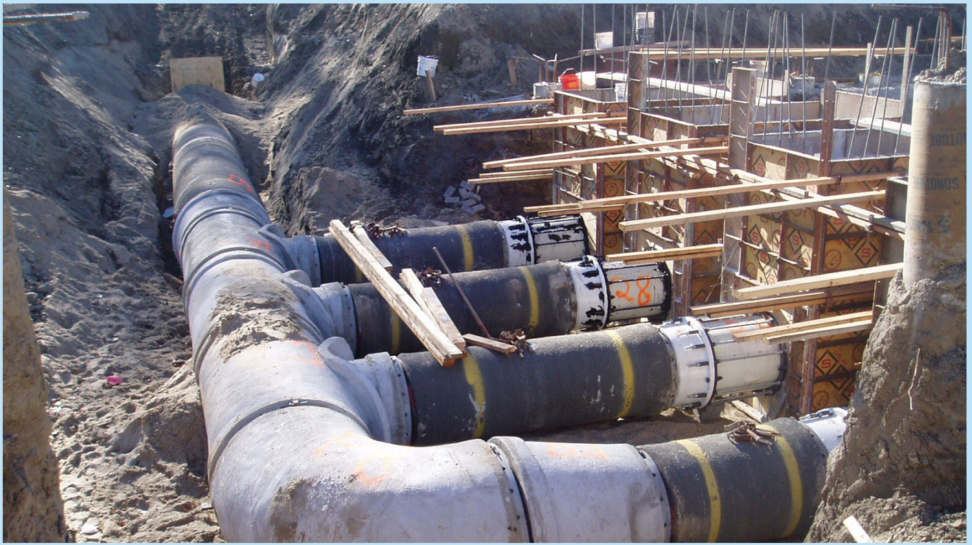
Concrete Pressure Pipe discharge header from high pressure pump station.
