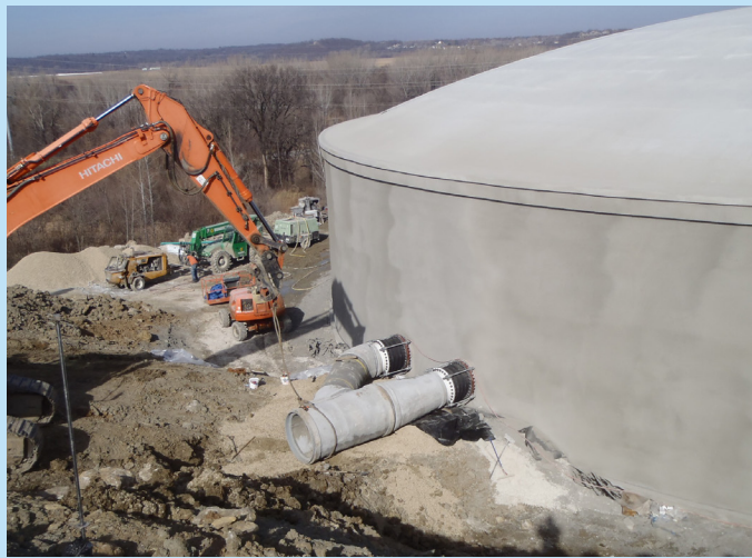
Concrete Pressure Pipe connects to treatment plant reservoir with flexible restrained joints.
